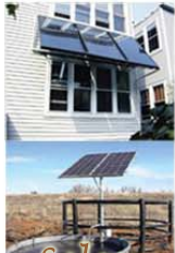
Solar PV Systems
